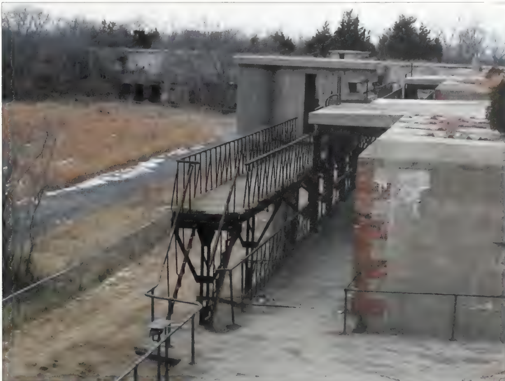
Figure 3.18. View looking west at battery commander's station Halleck, Nine Gun Battery. A cantilevered structure between emplacements #5 and #7, intended to provide access to the commander's station, is in poor condition (Olmsted Center, January 2009).
